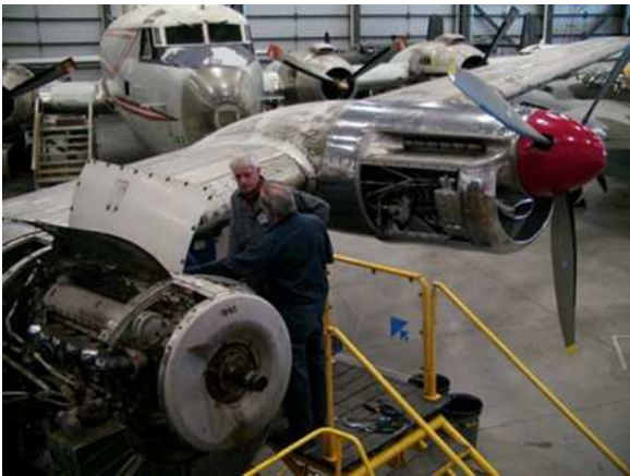
Figure 1: Jon Tasseron and Ted Devey prepare to remove the Nr 2 power plant. The fully restored Nr 1 power plant is on the right.
